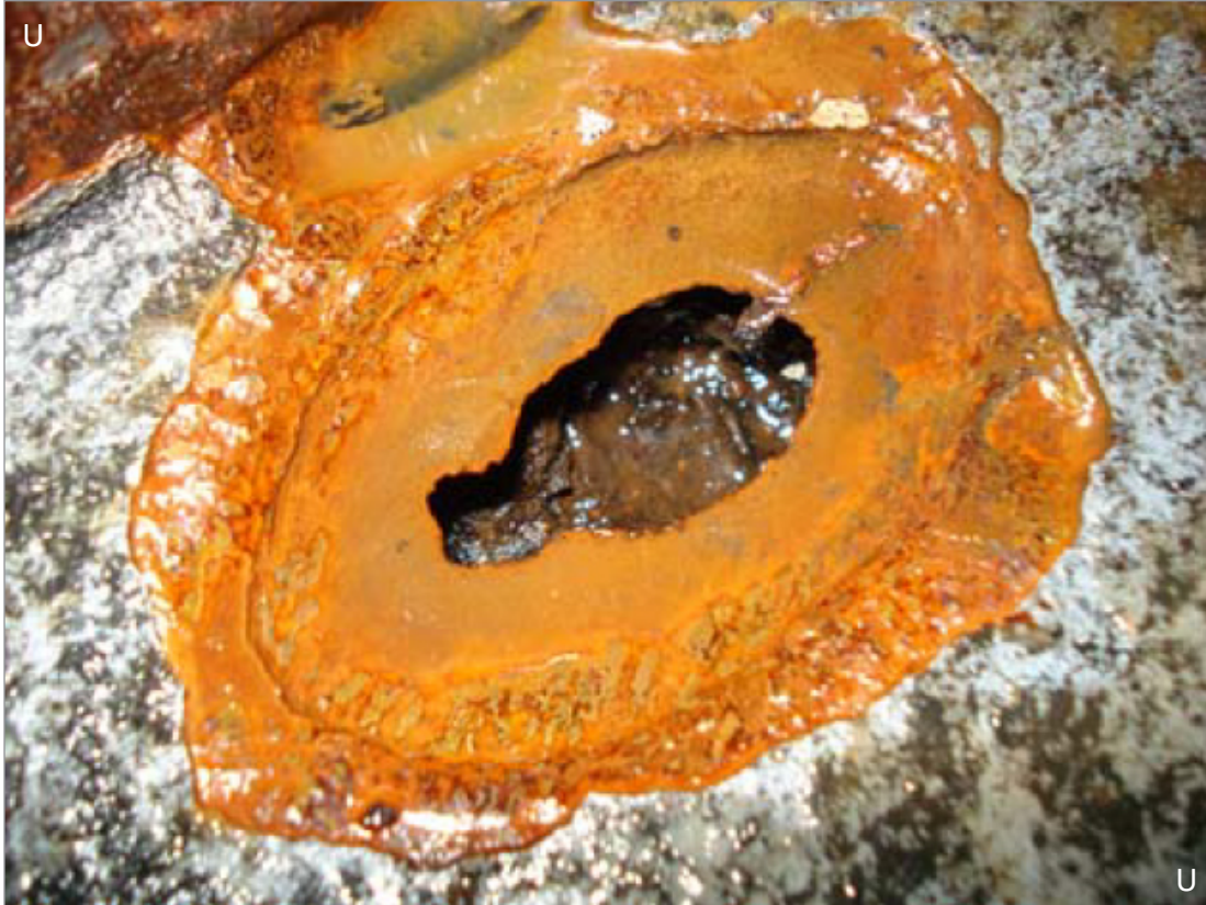
(U) Figure 9. Hole in Upper Tank Farm AST #48 at Naval Station Pearl Harbor (U) Source: NAVSUP.
